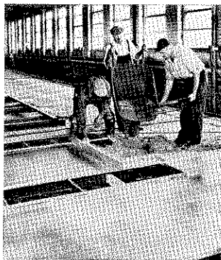
floor fill of perlite concrete can save tons of deadload in multi-story buildings.
